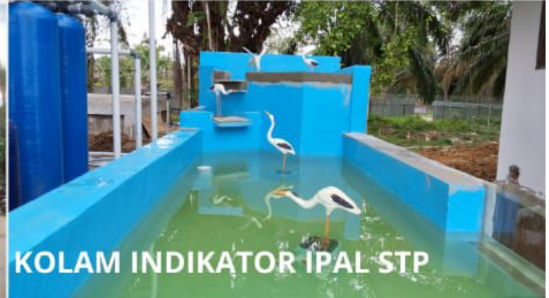
IPAL 1 STP (SEWAGE TREATMENT PLANT)
